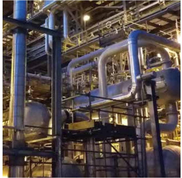
Industrial & Process Cooling Refrigeration
